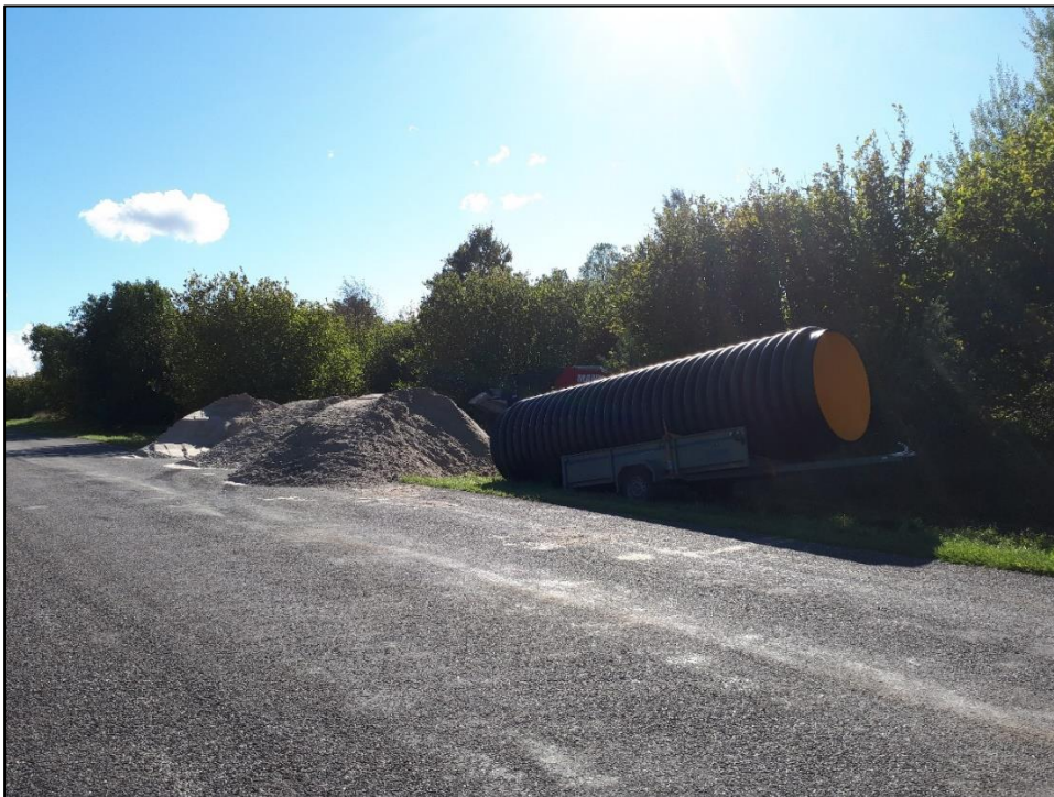
Photo 3. Culvert element and sand to be put on top of it waiting to be installed close to the vertical shaft in Vääna (Humala site). Photo by Lauri Klein
