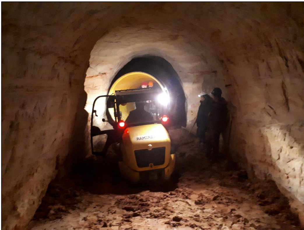
Photo 2. Installation of culvert element into rear tunnel of the Piusa largest cave system. Photo by Lauri Klein
